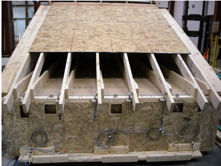
Figure 4 – Uplift set-up instrumentation (OSB panel is not attached to show connections and instrumentation)
