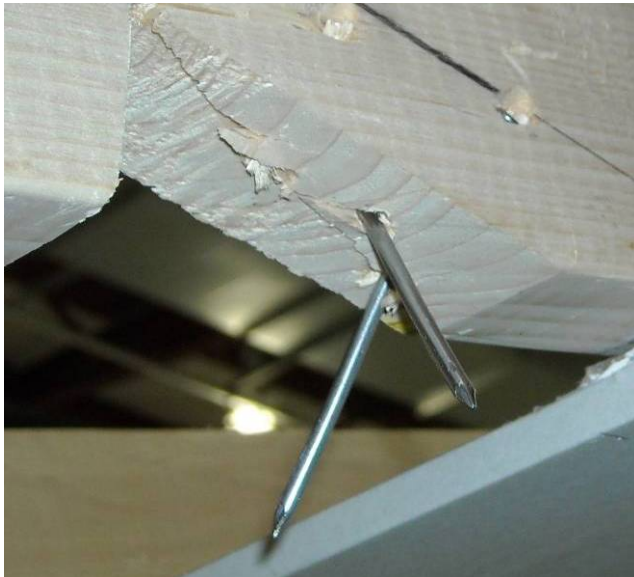
Figure 12 – Nail withdrawal and rafter splitting
